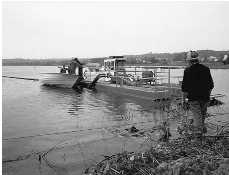
Figure 2 A cutterhead suction dredging machine 'Mudcat' used for dredging 500 000 m 3 sediment from shallow Lake Brabrand, Denmark.
